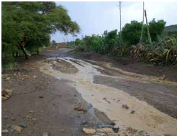
Unpaved roads often become drains
