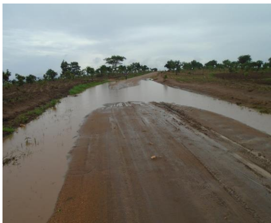
Condition of road before implementation
