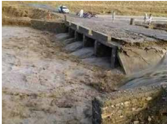
Figure 1: Example of vented bridge washed away by the force of the flood, Balochistan, Pakistan
