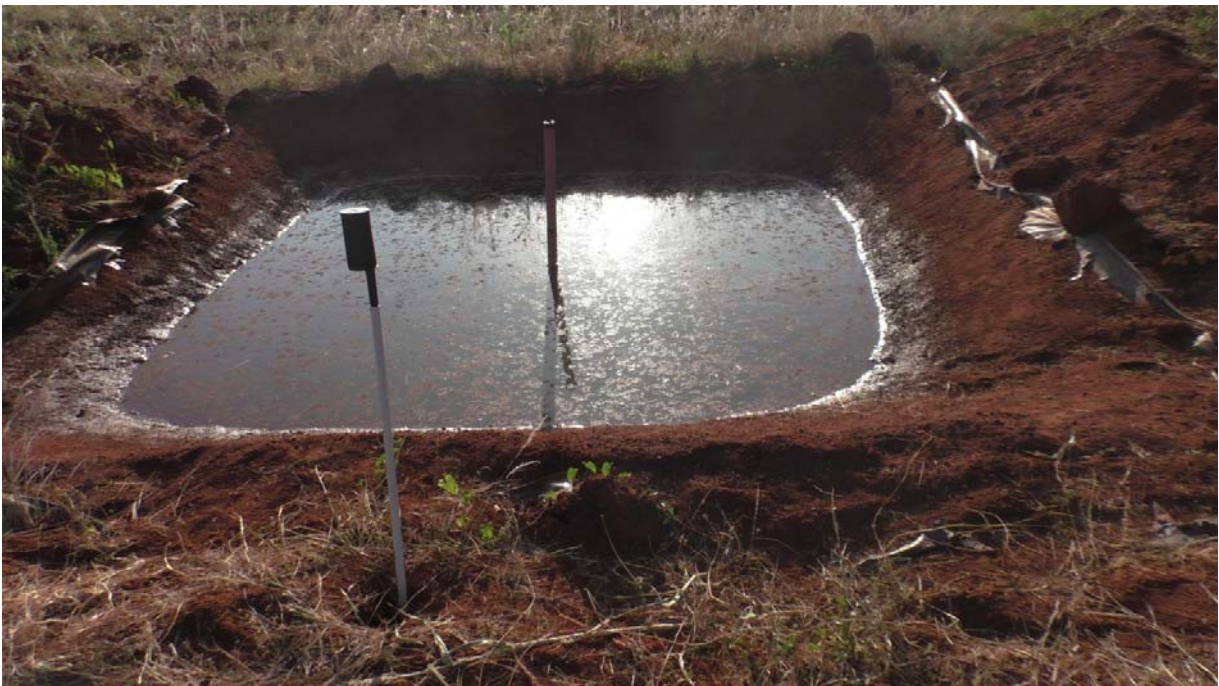
Figure 6: A pond lined with geomembrane and covered with field soil on top.
