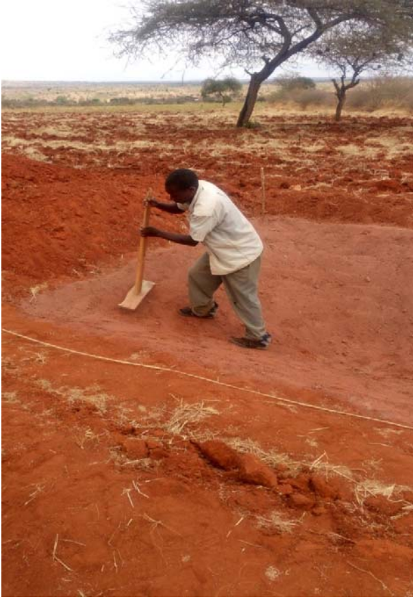
Figure 3: Compacting a mixture of soil and cement mixture layers applied on the pond size.
