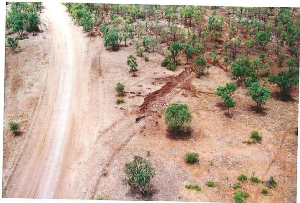
Plate 45. Poor siting of mitre drain discharging into a very active gully head.
