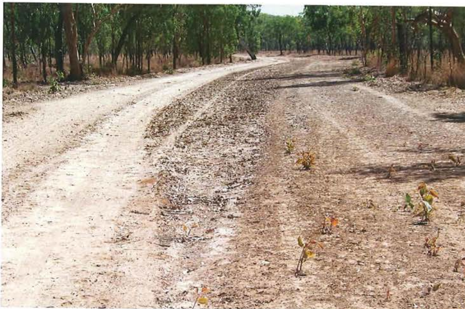
Plate 39. Poor site- boggy ground.
