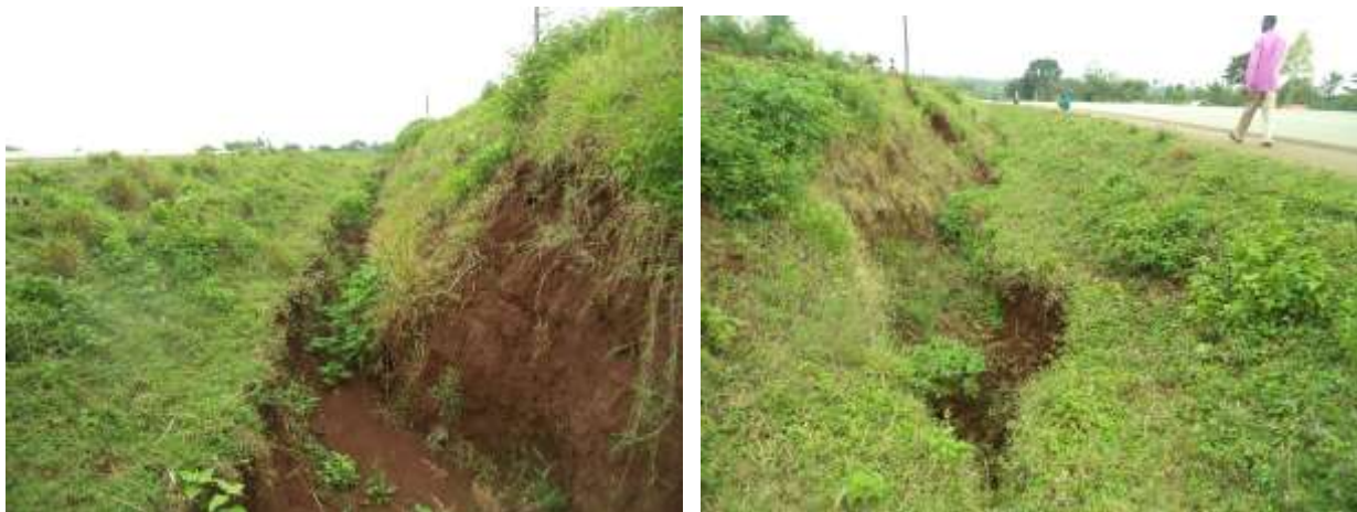
Figure 3-1 Gully formed due erosion along Tororo-Jinja Road in Busere village in Tororo District. (Threat of road collapsing)
