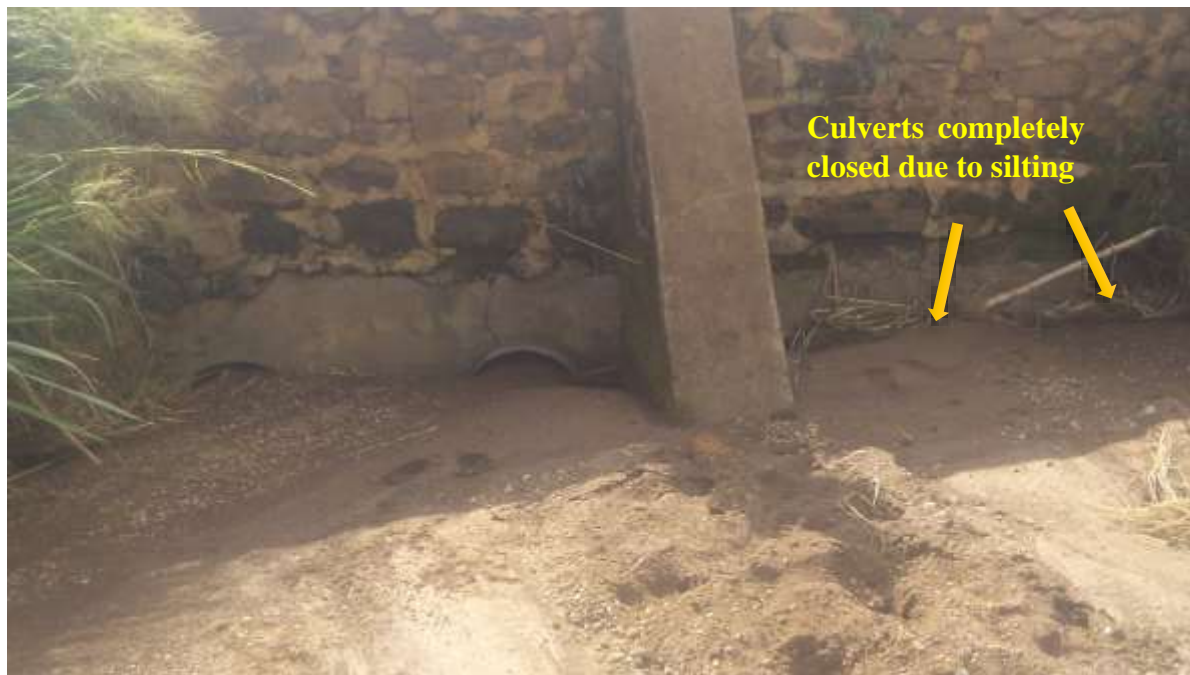
Figure 3-2 Siltation at Okurut Bridge located on the Road to Nakapiripirit District
