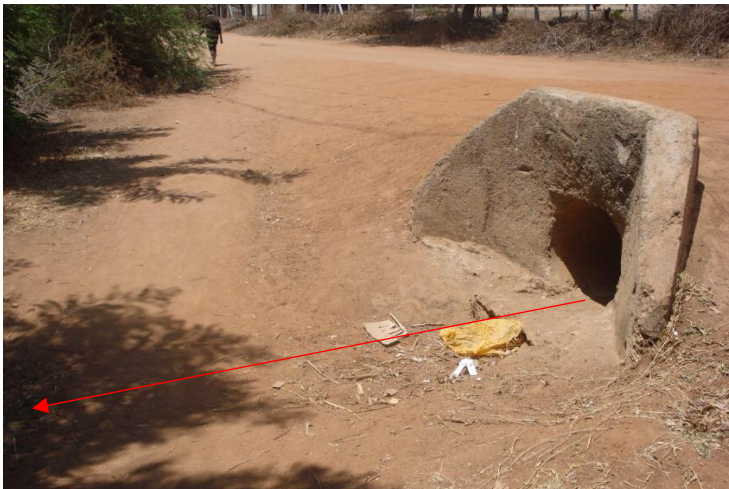
Figure 18: The outfall runoff
