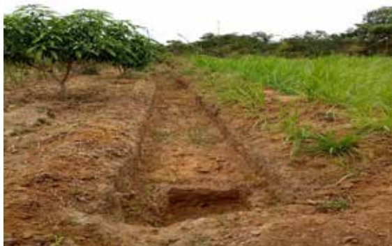
Figure 17: Retention ditch and terrace for conveying road runoff into the farm
