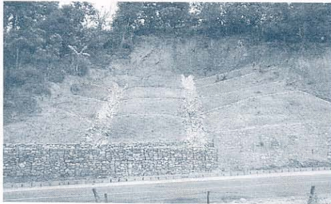
Stone-pitched surface drains on a wet landslide scar
