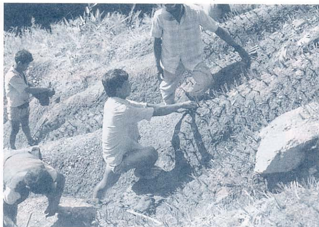
Grass planting on an eroded landslide scar. The supervisor is monitoring the works closely
