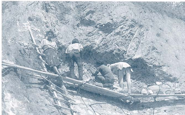
Constructing a cement masonry dentition wall to prevent undercutting of the upper part of a steep cut slope in differentially weathered gneiss
