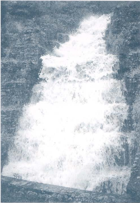
A gabion cascade in heavy rain. This type of structure can transport large volumes of water down steep slopes without damage
