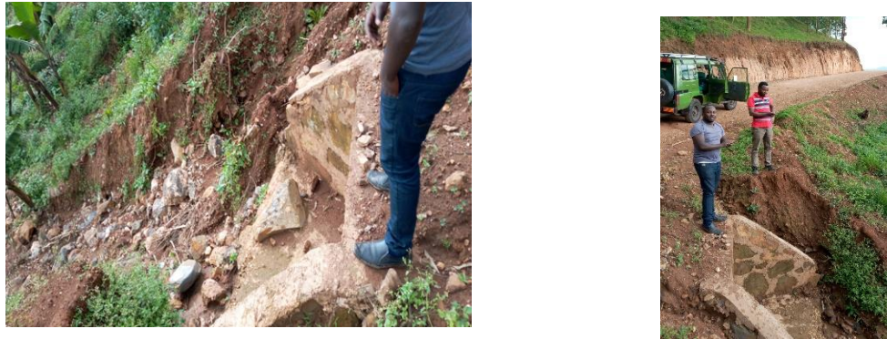
Figure 2-6 Erosion at culvert outlet
