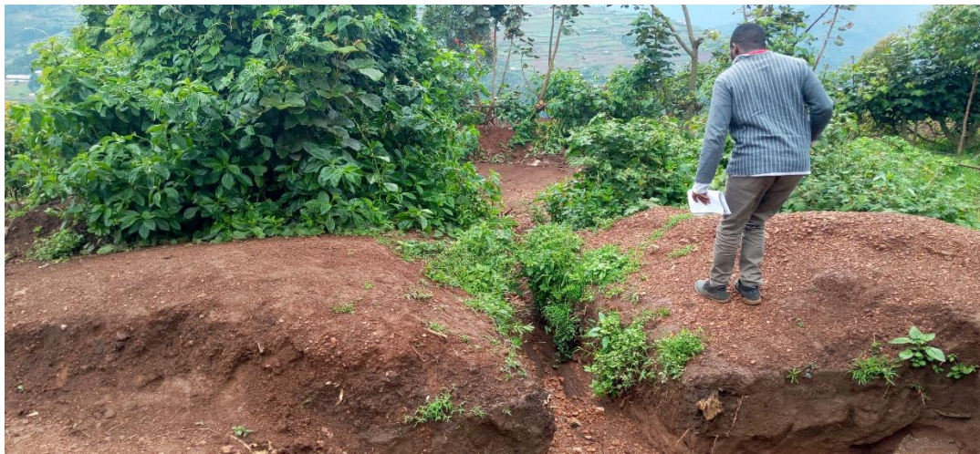
Figure 2-8 Silting at culvert outlet opposite Vision Primary School
