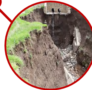
Erosion (gullies and landslides)
