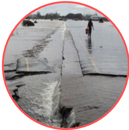
Water-related road damage (water causes 35-80% of road damage)
