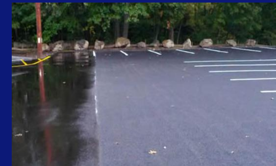
Porous pavement (right)
