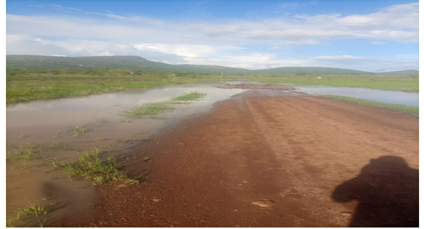
Flooded road section
