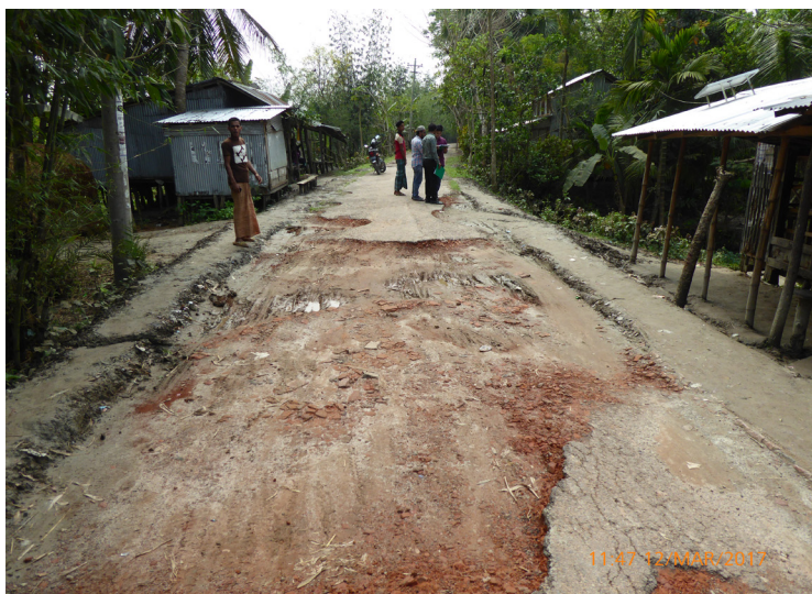
Figure 21: Poor quality embankment road.
